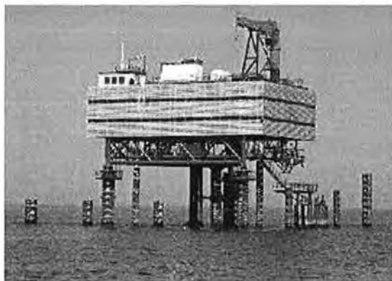
Figuur 2.12: Transformer Station, Horns Rev
