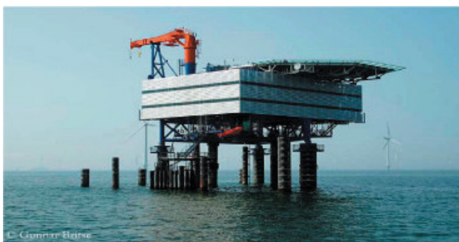
Figuur 2.11: Transformer Station, Horns Rev (courtesy Gunnar Britse)
